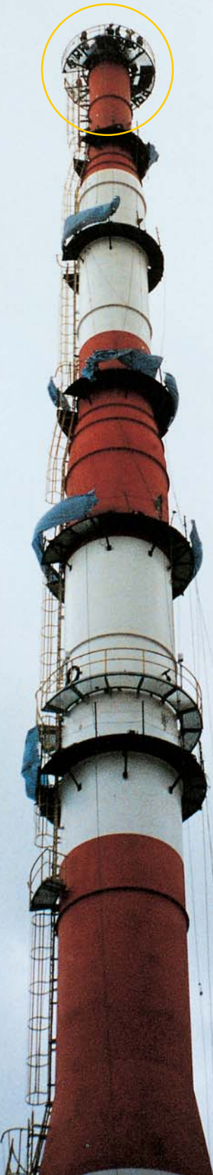
Chimney – Thailand (Ringdamper)
